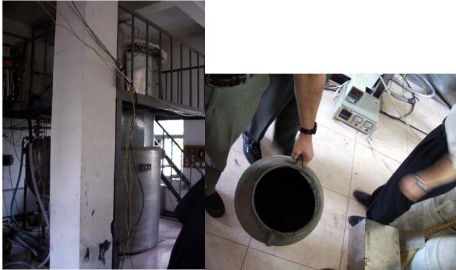
Figure B.26. 500 mm diameter FB reactor and entrainment separator.
